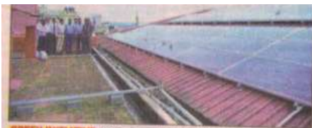
GREEN INITIATIVE: Rooftop solar plant installed at Yenepoya Medical College in Mangaluru on Wednesday
